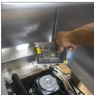
D1. Extract the defective power supply (secured on the tank's inner lining)
