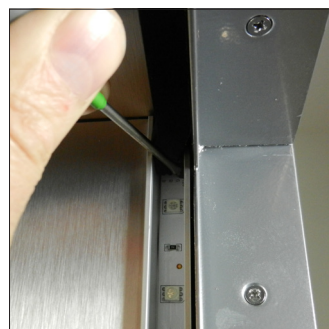
E2. Extract the broken LED strips from the guide, using a screwdriver
