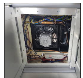
A5 . Condenser compartment
