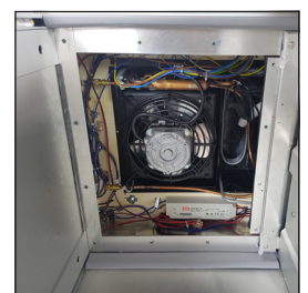
A5 . Condenser compartment
